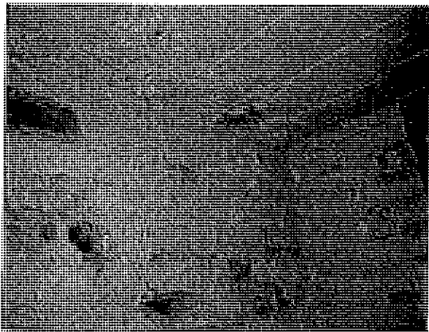
Figure 2: Evidence Room_Wet Exterior Wall
