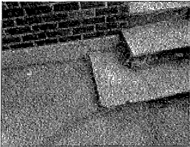
Figure 5: Damaged Concrete, Steps, Bricks
