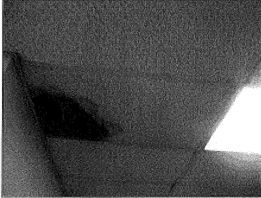
Photo 10: Leak in ceiling on 3 rd Floor from roof
