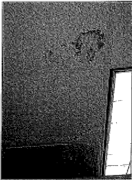
Figure 11: Electrical Hazard_Damaged Ceiling Tiles
