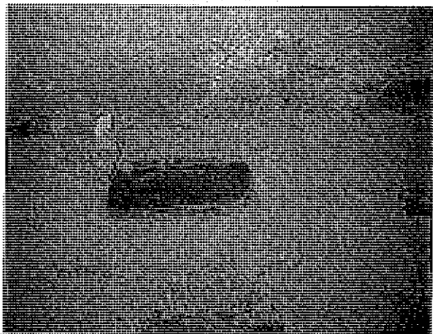
Figure 4: Evidence Room_Wet Falling Debris
