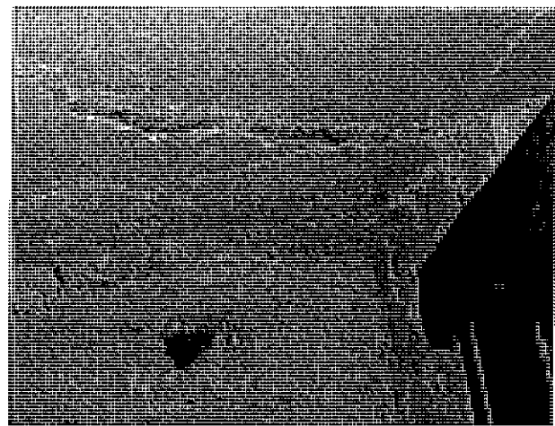
Figure 3: Evidence Room_Damaged Wet Wall
