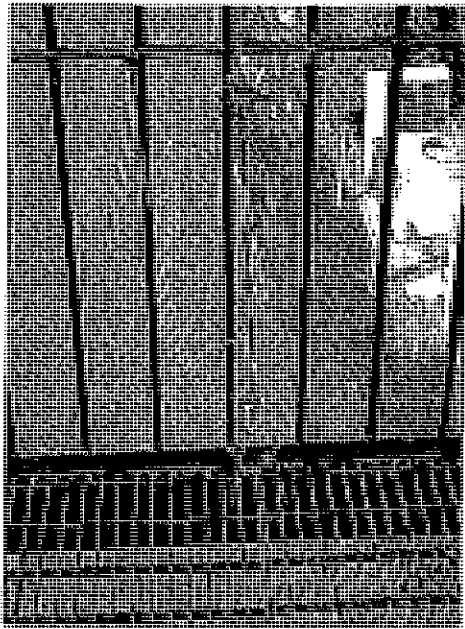
Figure 27: Fire Escape in disrepair
