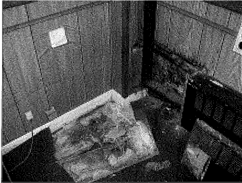
Photo 8: Example of mold on tiles and behind wall paneling in the Detective Room
