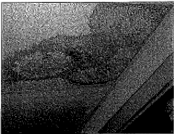
Figure 7: Mold_Damaged Ceiling Tiles
